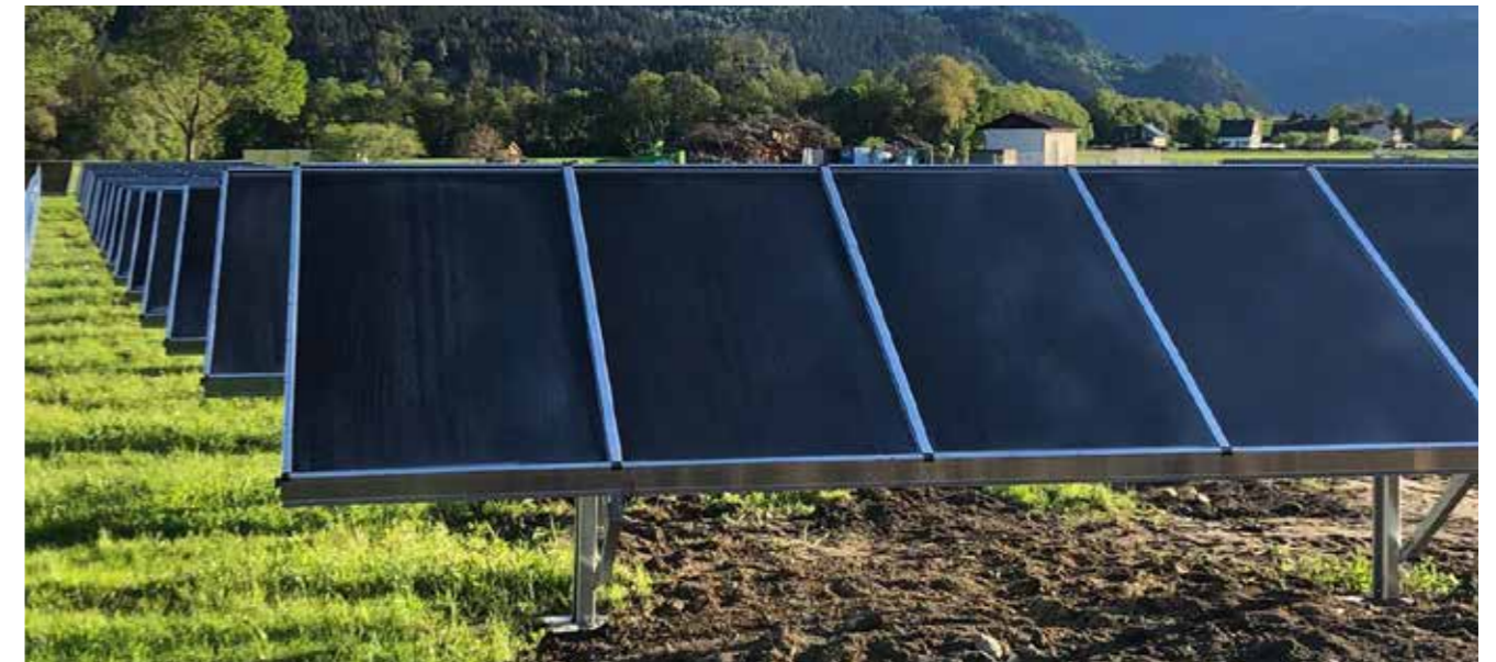
Solar thermal system Friesach
